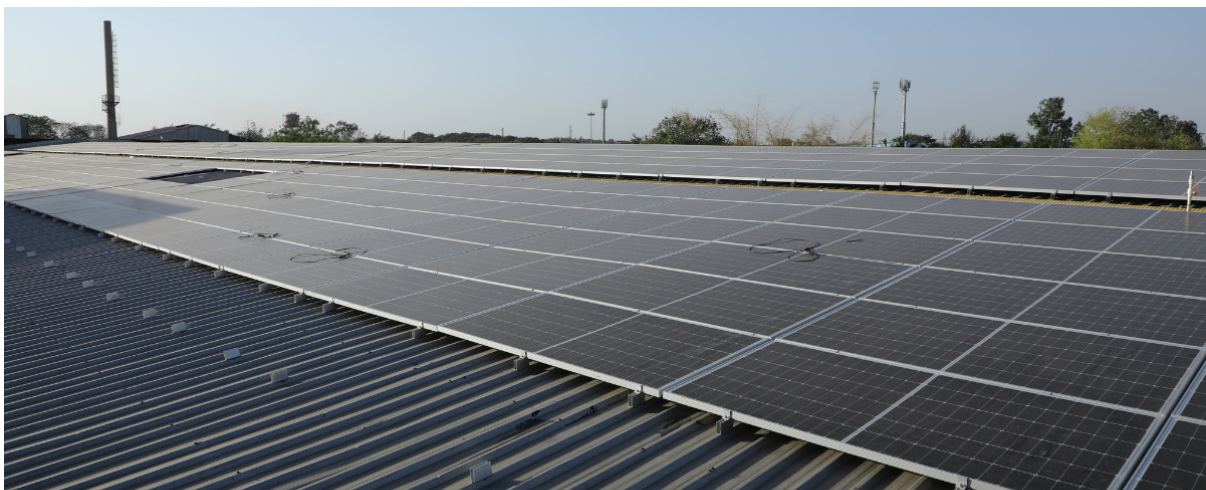
Rooftop solar panels at Pratibha Syntex
